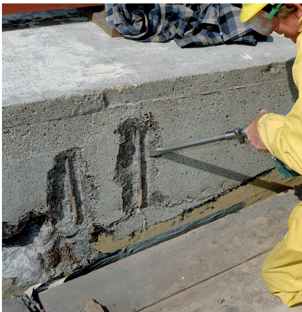
Damaged concrete structure
