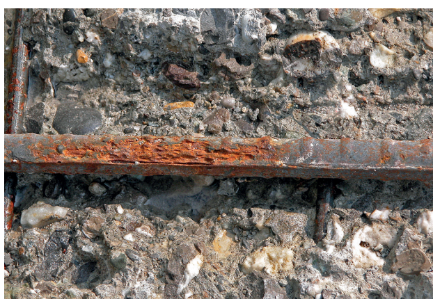
Damage to concrete structure due to insufficient concrete cover and low concrete quality.
